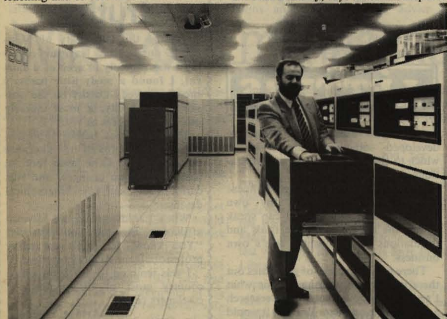
• "I know my lunch is in one of these drawers..." Computer Centre Operations Supervisor, Brian Potton, changes a disk pack in Monash's newly-installed B7800 computer. This picture shows only about a third of the main installation, which occupies a room 17m by 13m. Photo: John Keesing.
