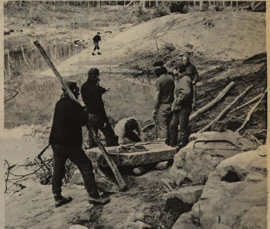
MUSCLE-POWER was needed at this stage of the operation. Moving the heavy slabs of rock from their resting place to the makeshift helicopter pad 200 yards away took the work party about a day and a half.
