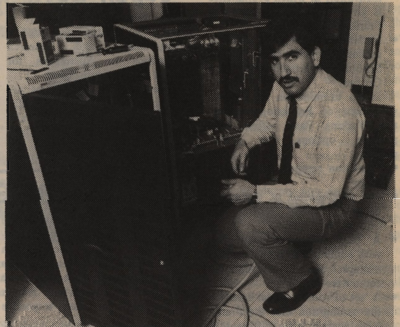
Installation of the Centre's new Digital VAX 11/750 central processor has completed in June. Digital field service engineer, Mr Bambos Haralambous is pictured doing some fine tuning.
